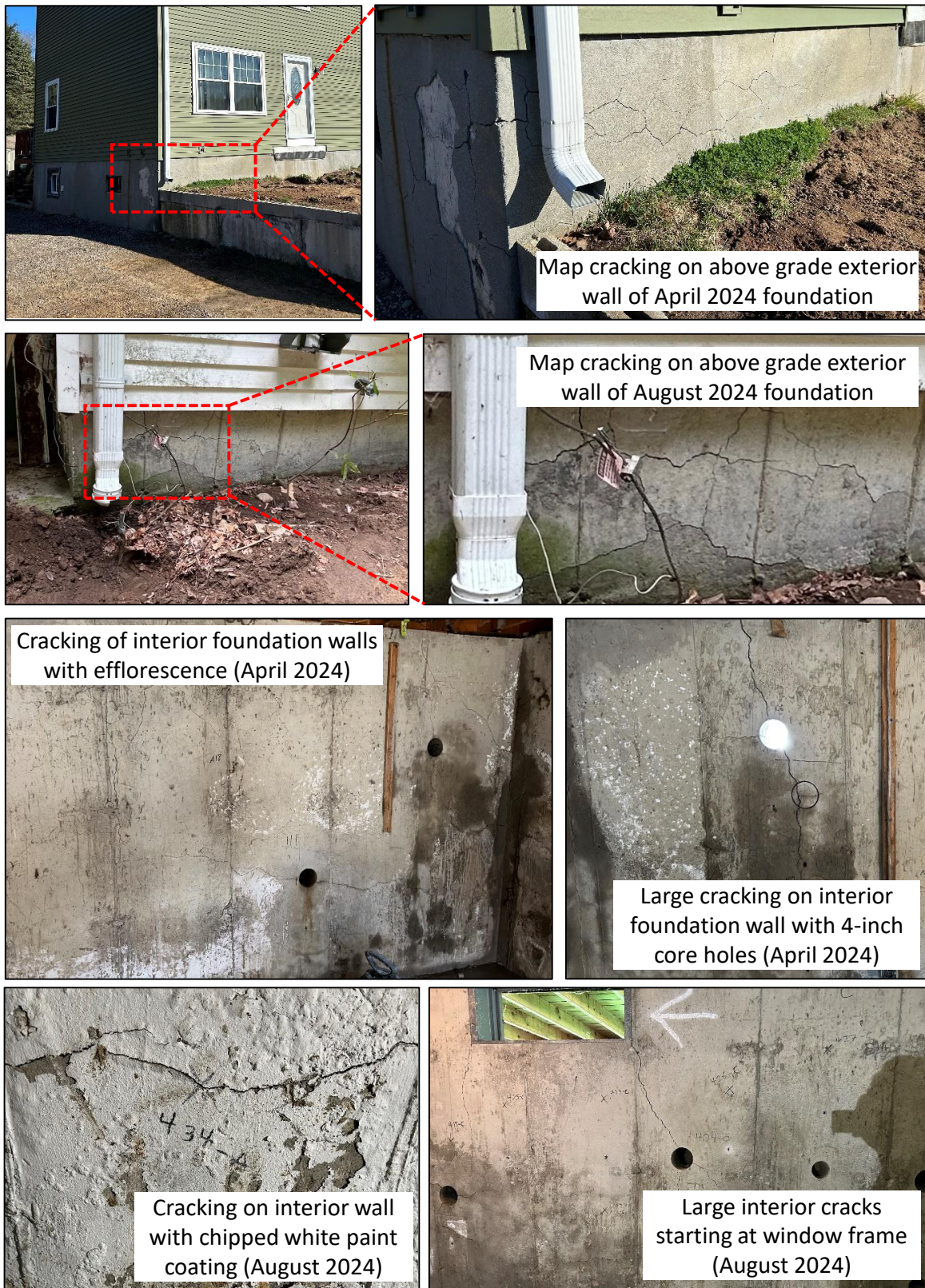
Figure 1. Photographs of deteriorated foundations sampled by NIST personnel in April and August 2024 detailing the level of damage typically seen in foundations prior to replacement and removal
