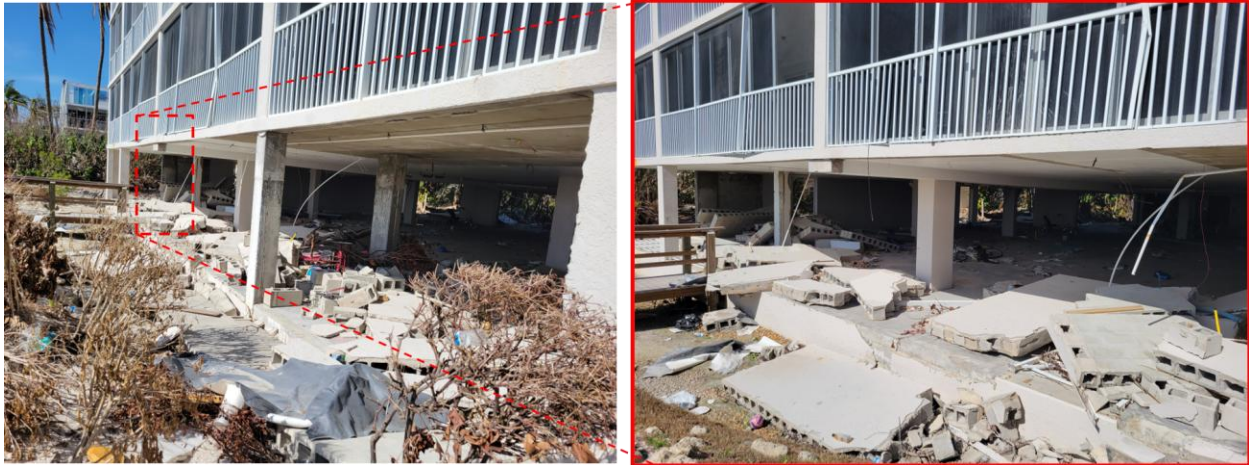
Figure 7. Failed column without collapse.
