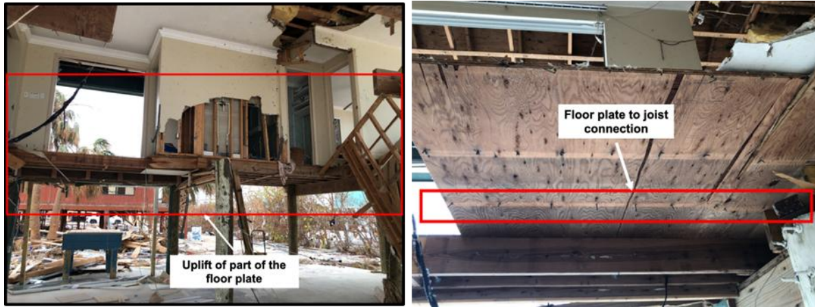
Figure 5. Severe structural damage to the elevated floor and balcony of a wood-frame house due to the hydrodynamic wave uplift force.
