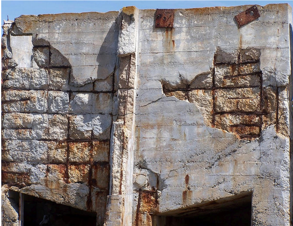
Fig. 2. Severe corrosion damage in an abandoned steel-reinforced concrete structure on McAbee Beach in Northern California; adapted from [2].
