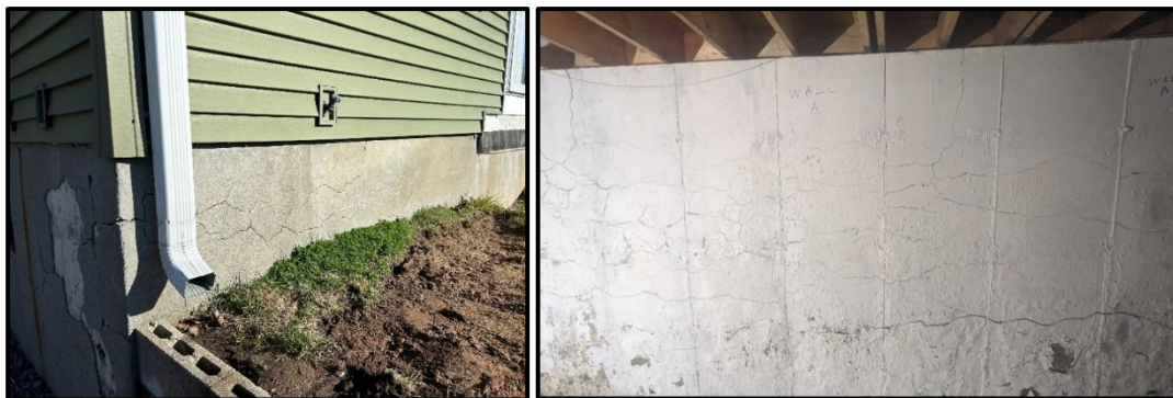
Figure 1.1: Deterioration of concrete foundation due to pyrrhotite
