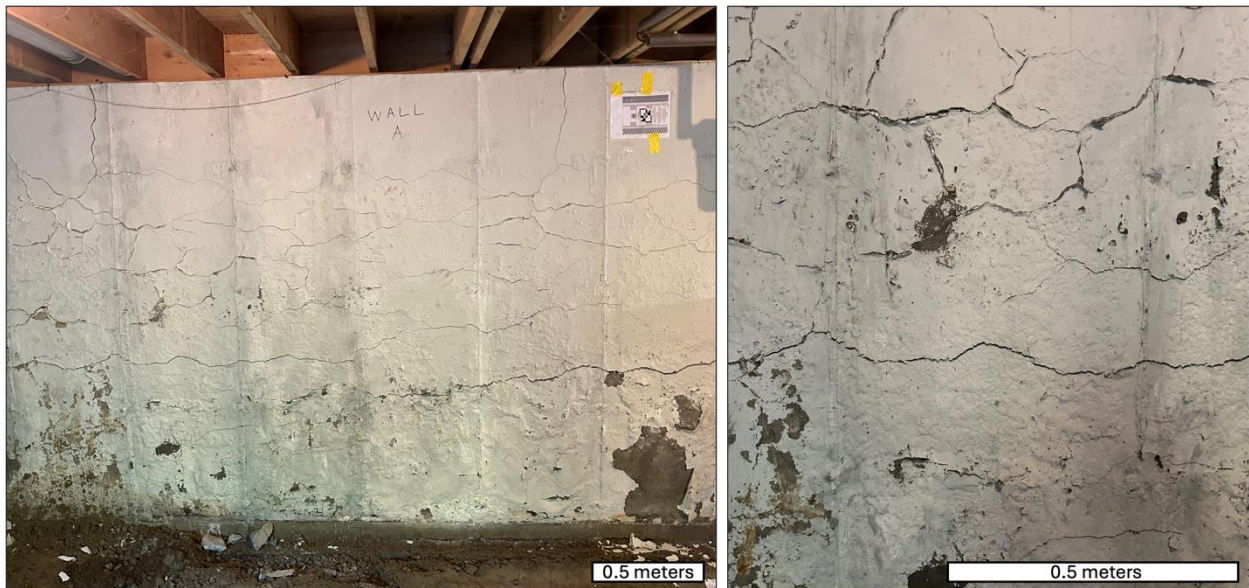
Fig. 1 Map cracking in a residential foundation sampled during a NIST field study. Images of a residential foundation slated for removal and replacement showing extensive intersecting fractures termed “map cracking.” [Photo Credit: NIST]
