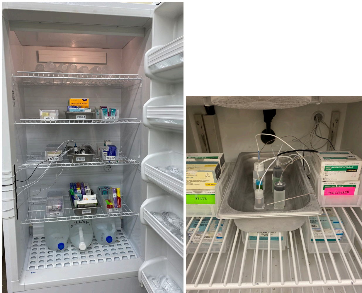
Fig. 7a, 7b. DDL installation in a standalone refrigerator (left) and an undercounter freezer (right).
