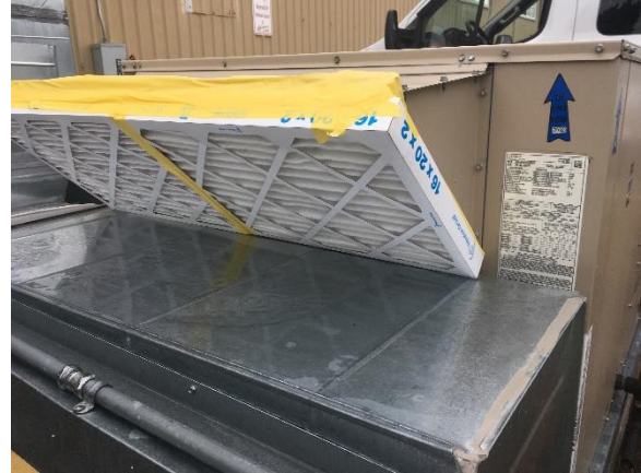
Figure 4. Picture of a MERV 13 filter installed on an intake air vent
