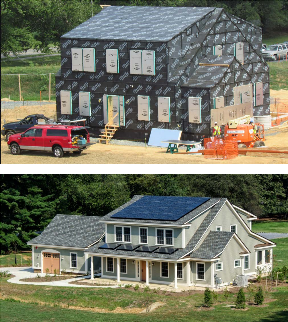
Figure 1. Construction of NZERTF showing the air barrier (top) and completed structure (bottom).
