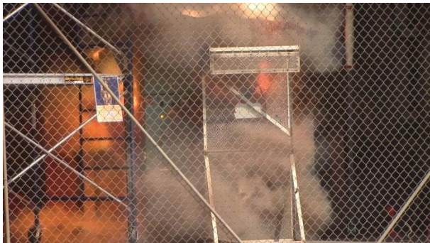
Figure 9 Low voltage HEAF; front of cabinet
