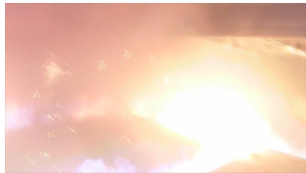
Figure 10 Low voltage HEAF; top of cabinet; cable tray visible in upper right of photo
