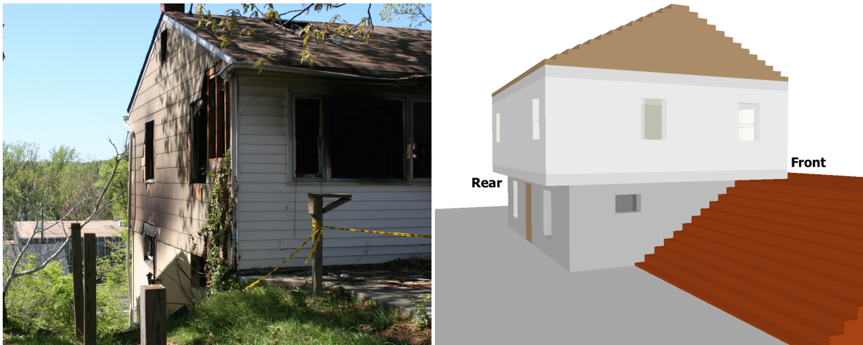
Figure 3.1: Photograph taken from front side street level showing the slope down to basement on the rear side of the structure (left) and Smokeview rendering of model representation of sloped landscape (right).
