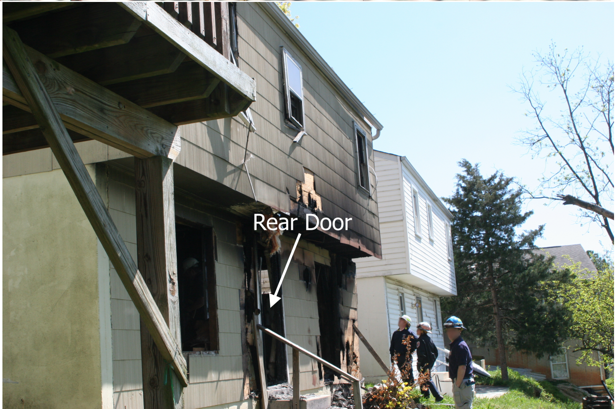
Figure 3.3: Photographs showing the front (top) and rear (bottom) exterior of the structure after the incident.
