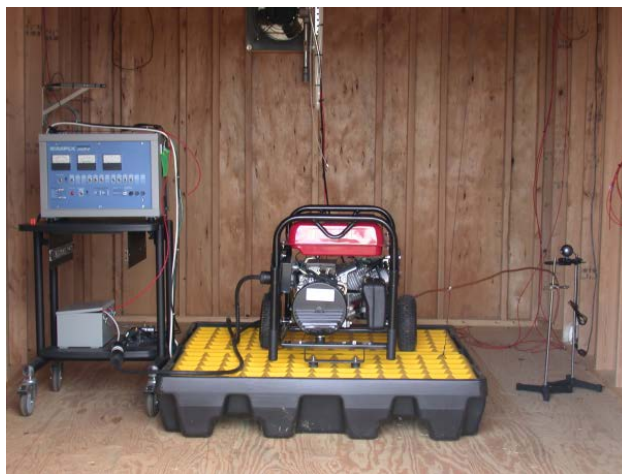
Figure 2. Generator in test shed
