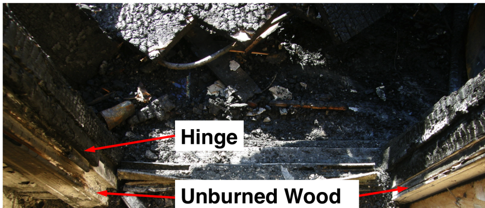
Figure 3.3: Post-incident image of the second floor porch door frame that failed taken from inside the structure looking toward the porch. Note that the hinge is still intact and there is unburned, “clean” wood along the bottom portion of the frame.
