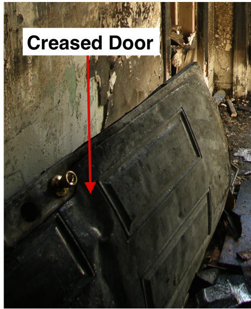
Figure 5.1: Post-fire image of interior door.
