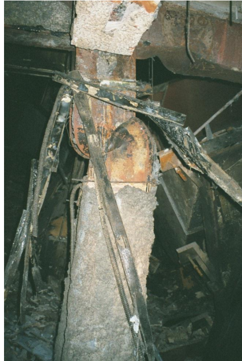
Figure 14. Buckled column on the 8 th floor of WTC 5 (photograph from FEMA 2002).
