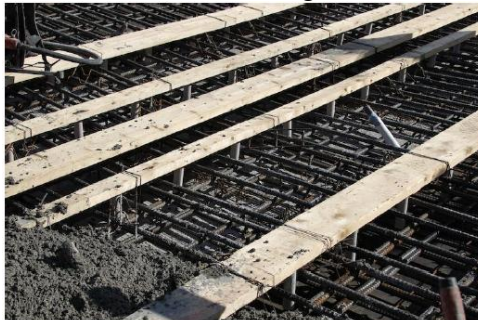
Figure 1: A railway bridge deck rebar cage with the dowels and wooden planks installed [Saidi, K., et al., 2011].
