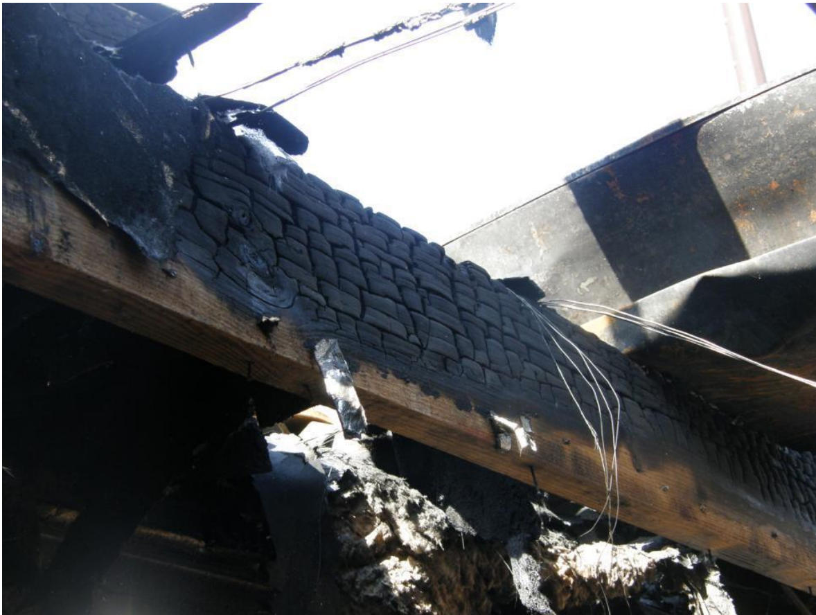
Figure 6: Charred rafter located above the dining room
