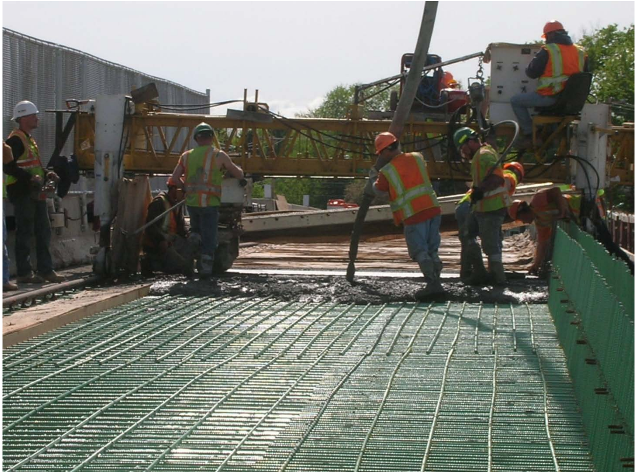
Figure 45. Internally cured concrete being cast at Bartell Road in New York (Wolfe, 2010).
