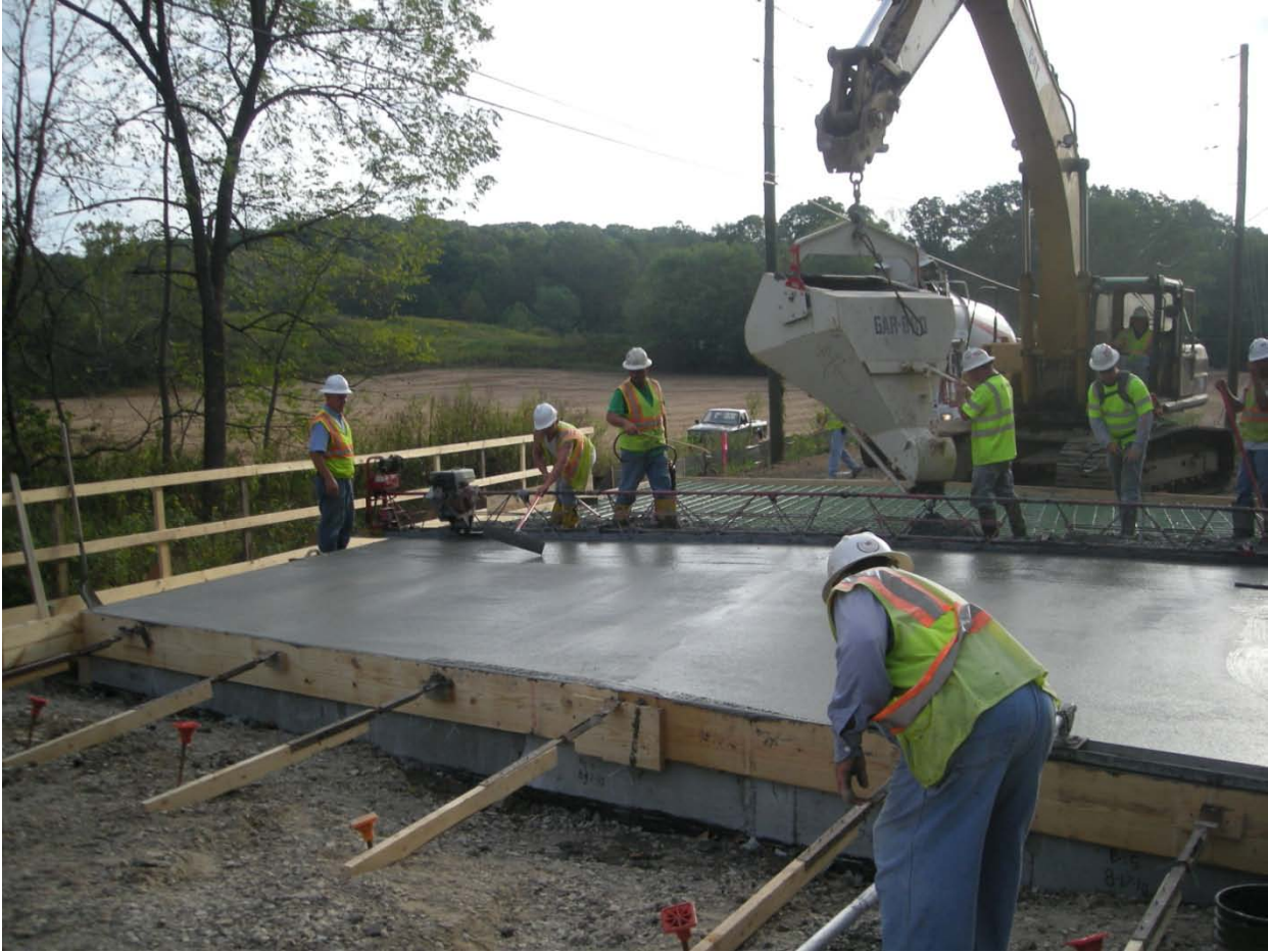
Figure 46. Internally cured concrete bridge deck being cast near Bloomington, IN (Di Bella, Schlitter, & Weiss, 2010).
