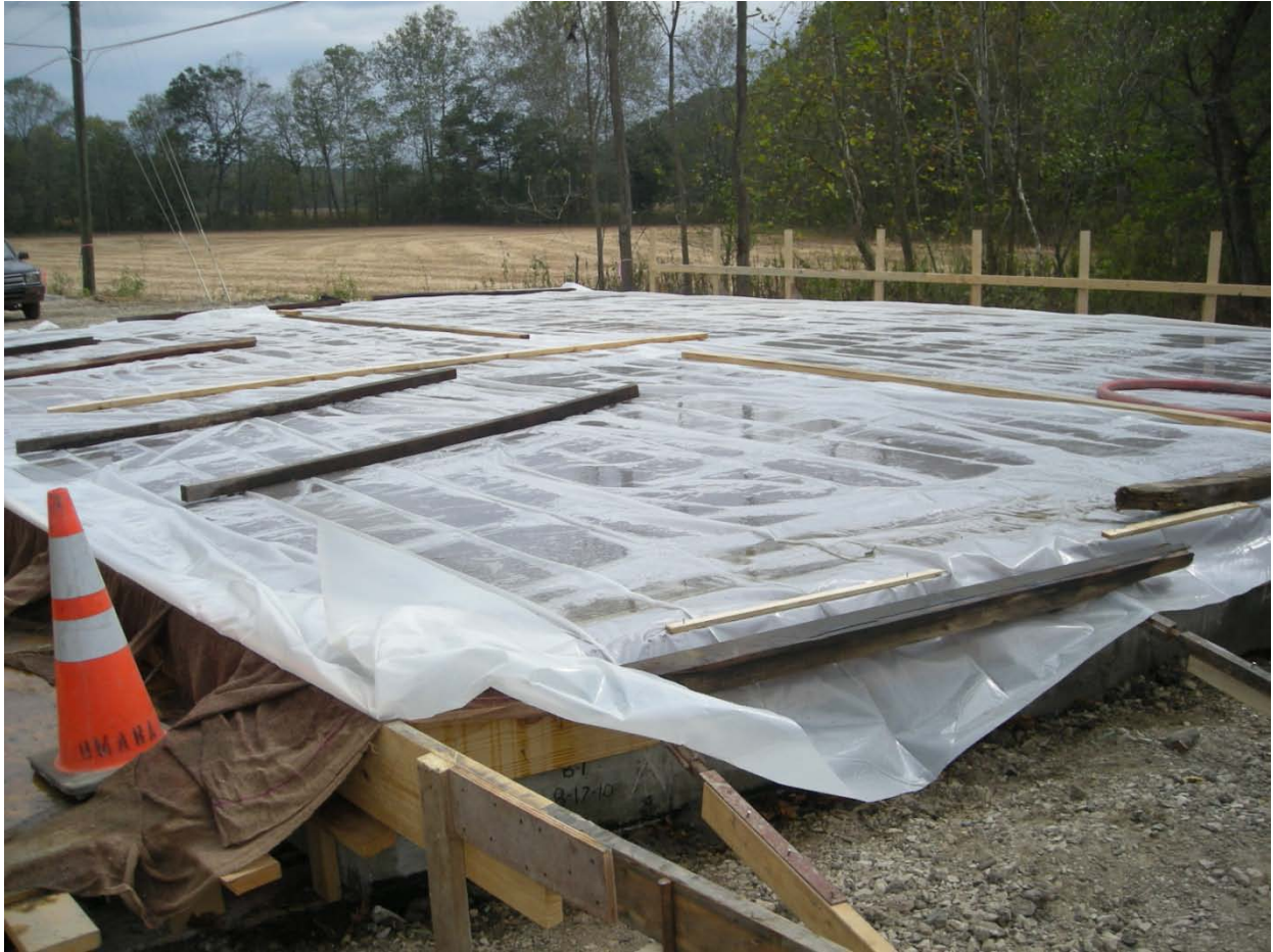
Figure 48. Plastic sheeting being used to cover the wet burlap on the internally cured concrete bridge deck near Bloomington, IN (Di Bella, Schlitter, & Weiss, 2010).
