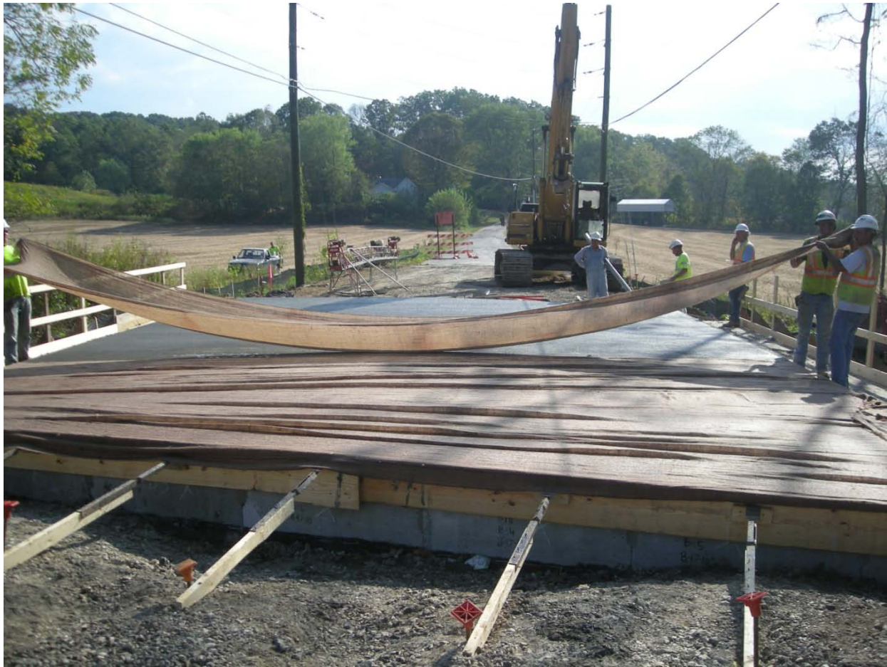
Figure 47. Wet burlap being used on the internally cured concrete bridge deck near Bloomington, IN (Di Bella, Schlitter, & Weiss, 2010).
