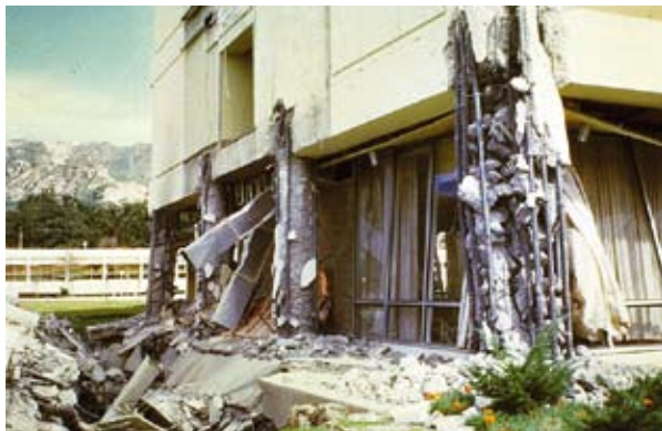
Earthquake damage to the Olive View Hospital in San Fernando, CA, from the 1971 earthquake.
