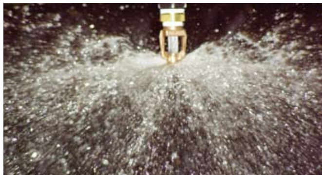
A close-up of an activated fire sprinkler.
