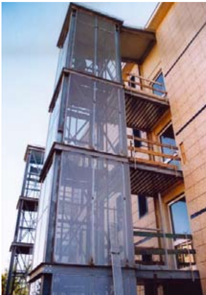
This smokeproof elevator is installed at an Italian residential facility for mobility impaired people to provide access and egress. The glass hoistway enclosure permits the fire service to determine if the elevator is in use. (Photo courtesy of the Italian National Research Council)
