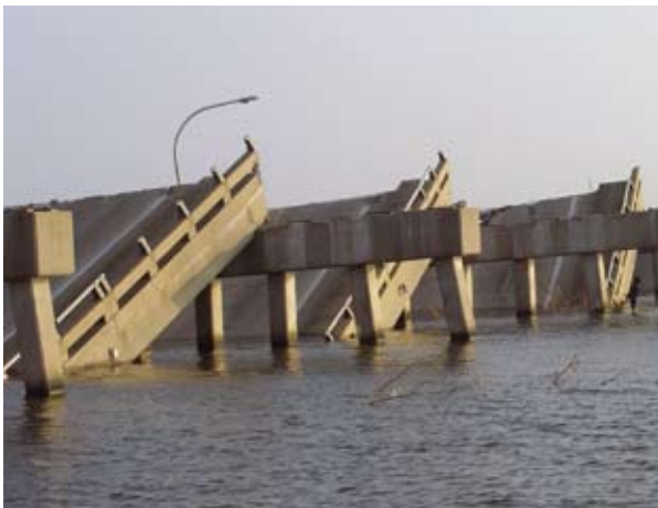
The US-90 Biloxi-Ocean Springs bridge (looking west toward Biloxi from the east shore). Simply supported superstructure spans were displaced and dropped north off their piers due to storm surge and wave actions during Hurricane Katrina in 2005.
