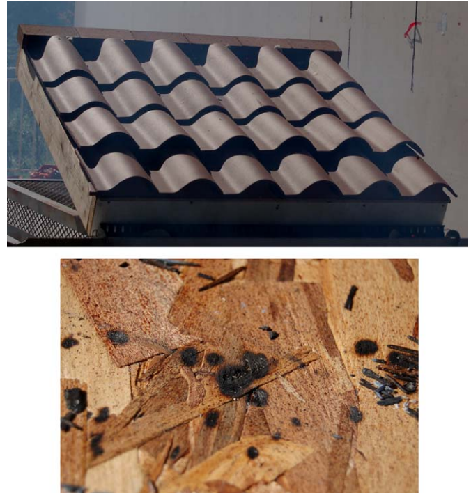
Fig. 11. Images of ceramic tile roof assemblies purposely constructed with gaps within the tiles. Multiple SI observed with OSB base layer.
