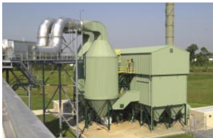
Newly installed pollution abatement system for the Large Fire Laboratory.
