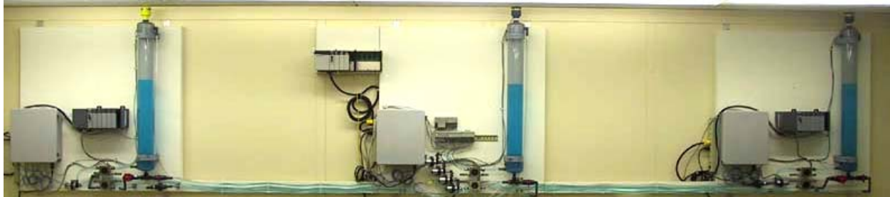
Figure 4 Water distribution SCADA system
