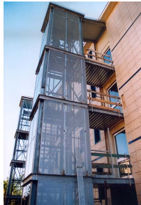
This smokeproof elevator is installed at an Italian residential facility for mobility impaired people to provide access and egress. The glass hoistway enclosure permits the fire service to determine if the elevator is in use. (courtesy CNR)
